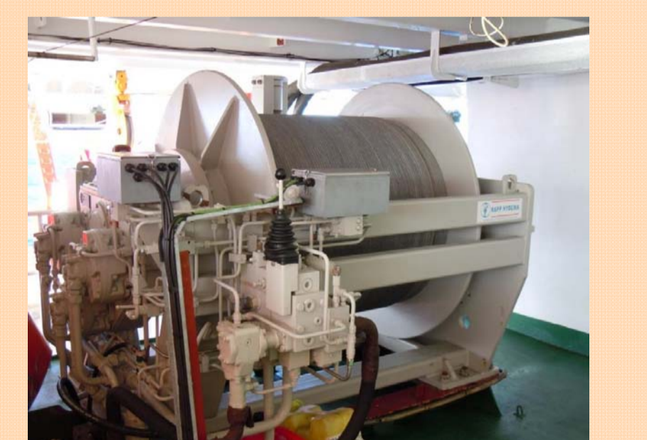
New winch installed, 11 mm dia. cond. Cable 8000
